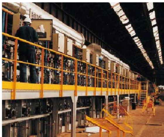
Fig 6. Multi burner oven application
